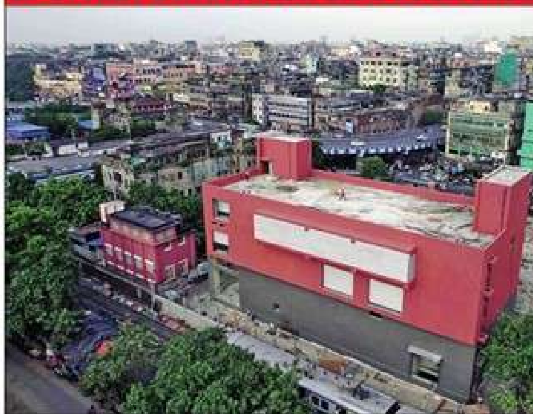
The ventilation-evacuation shaft at the Strand Road riverside
