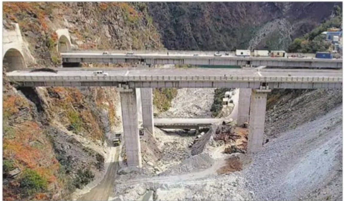
A view of the Kiratpur-Manali four-lane road from Pandoh to Takoli. PHOTO: JAI KUMAR
