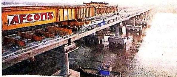
The last span of the Kasheli Creek Metro viaduct was erected on Sunday. Express
