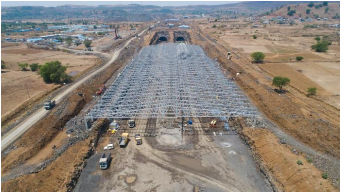
The tunnel is 7.78 km long, in two tubes with a total width of 35 metres — 17.50 metres in each tube. Credit: Special Arrangement
