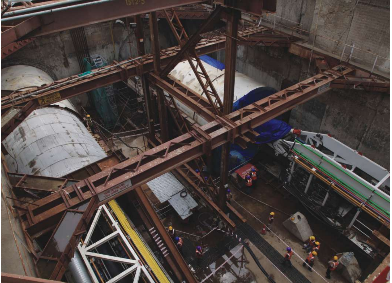
Tunnel Boring Machine (TBM) launch at Chennai Metro Rail Site on 28th December 2012
