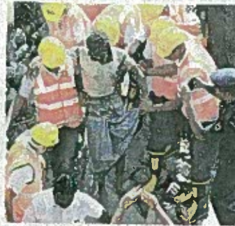
NDRF, fire services and CMRL personnel swung into action to rescue workers trapped at the accident site
